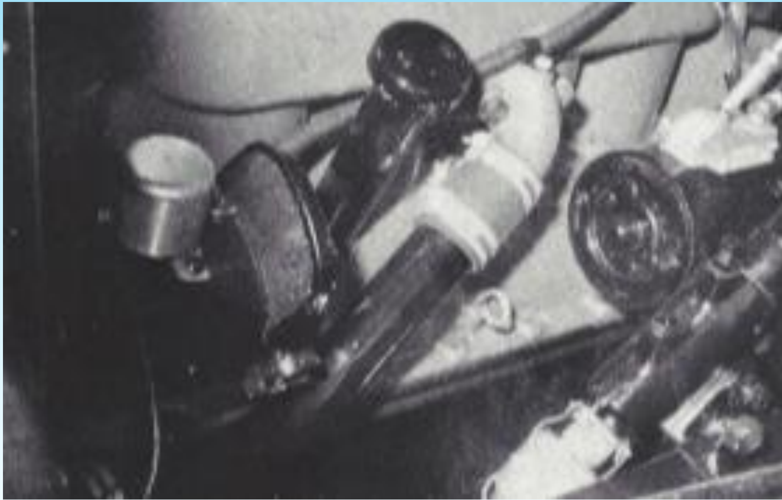
Generator Air Scoop and Filter
